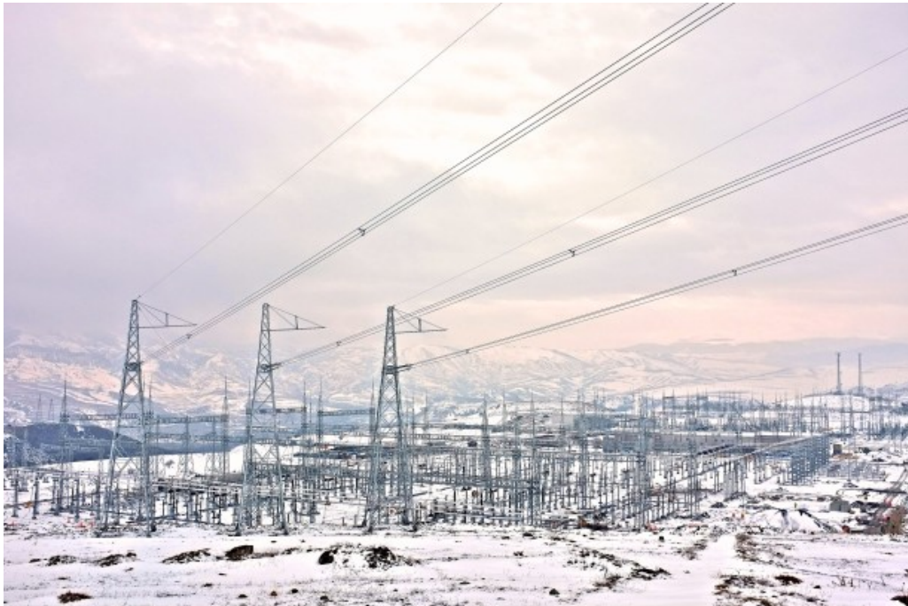
The new transformer substation. Source: Elmar Neubauer
